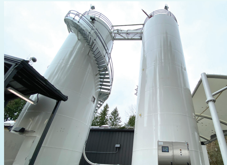
Improved Corrosion Control Treatment facility
